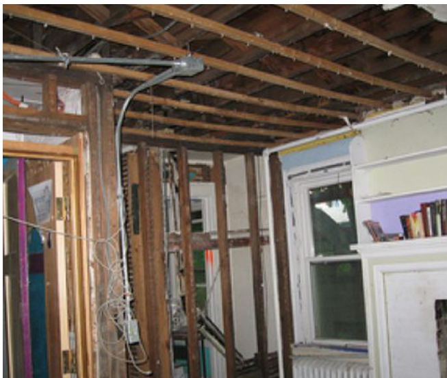
Photo of existing building interior showing where new walls and ceiling are required
